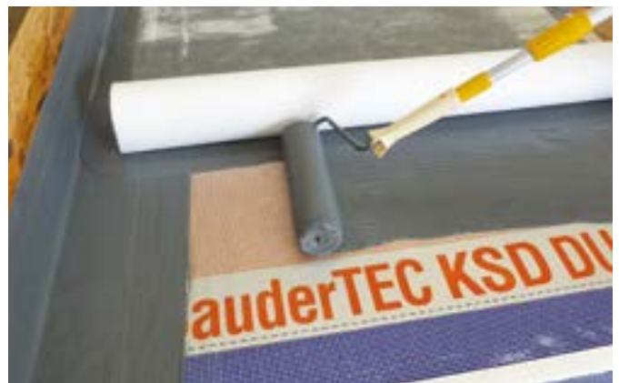
No.5: LiquiDEK is applied over the carrier membrane and the reinforcement fleece is rolled in..
