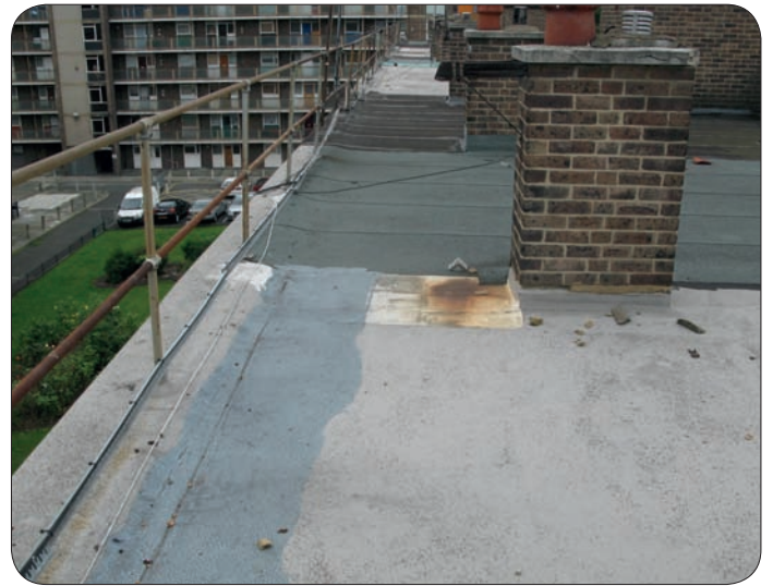
Daytime observation of a roof area at Shaftesbury Court with no apparent signs of water ingress.
