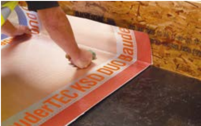
No.1: Air and vapour control layer installed to primed substrate, terminating 100mm past the surface level of the proposed insulation.
