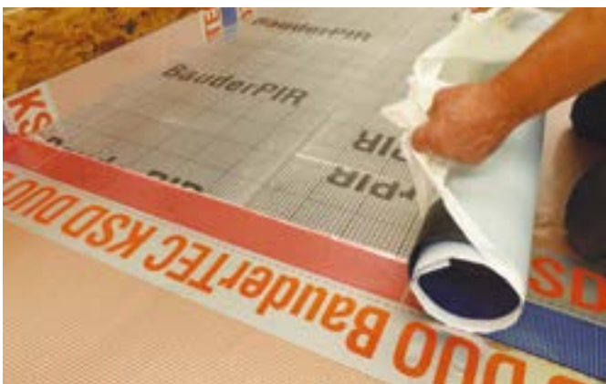
No.3: Carrier membrane installed over the insulation, lapping with the AVCL at details by 50mm.
