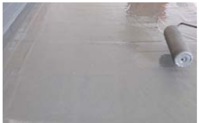
No.6: A further coat of LiquiDEK over the reinforcement fleece wet-on-wet completes the installation.
