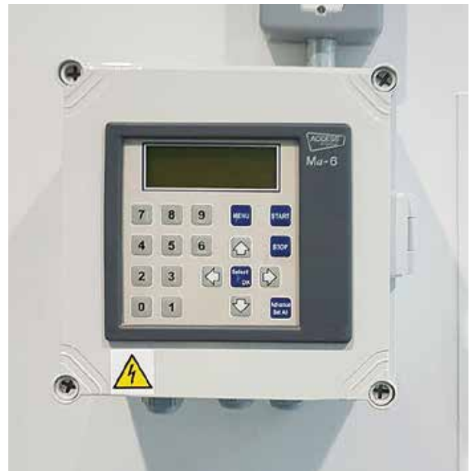
▲ An example of a wall mounted control box used in conjunction with an automated irrigation system
