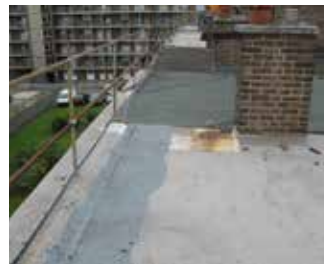
Daytime observation of a roof area at Shaftesbury Court with no apparent signs of water ingress.
