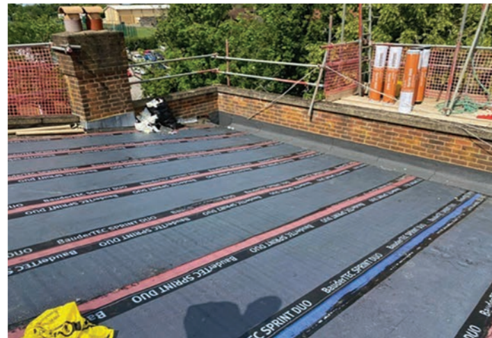
A solar photovoltaic (PV) array had been installed on one side of the roof and the rails it was mounted on had been screwed directly into the roof deck through the membrane, creating numerous points of penetration.
